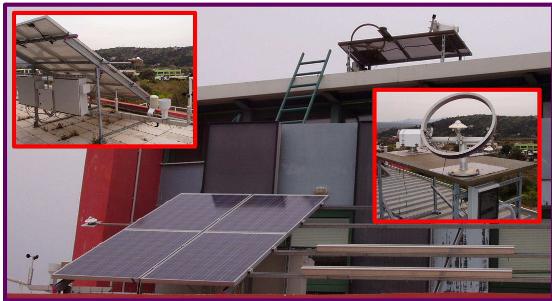
Fig. 1 Long-term test of PV modules
